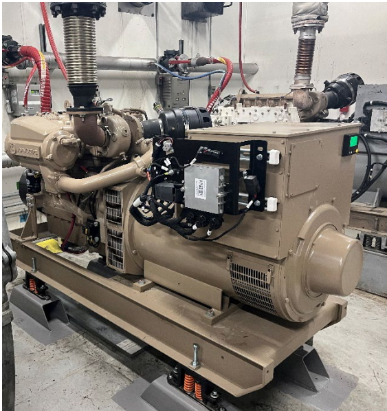
Existing Gen#2 (Gen#1 Behind)
