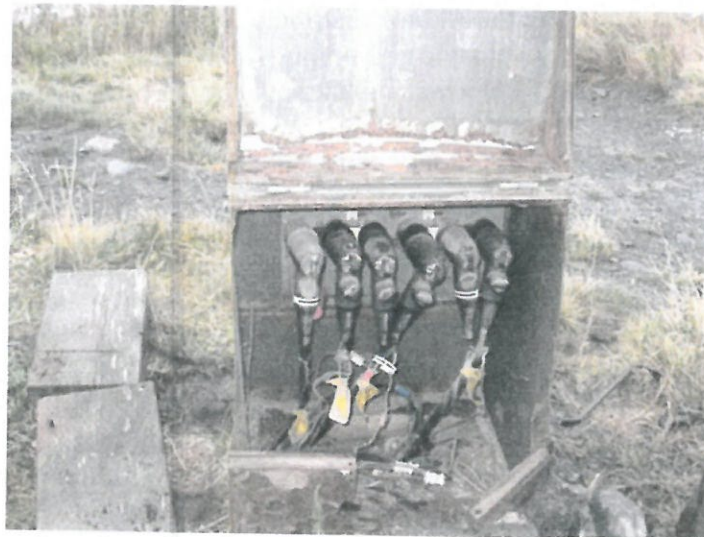
Figure 12 – Rusted Junction Box #4
