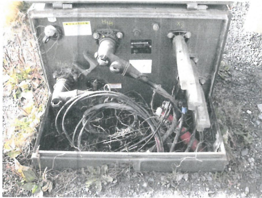
Figure 14 – Health Clinic Transformer
